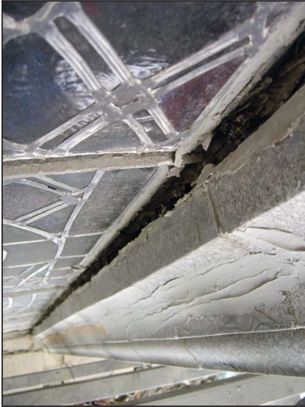
A window reglet or groove in poor condition.
