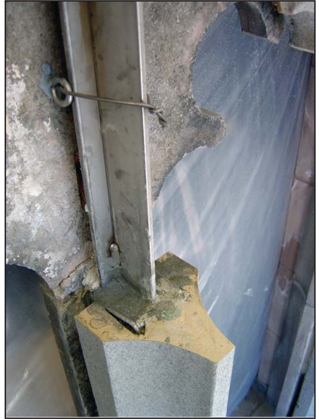
The installation of a new stainless steel "T" mullion and terra cotta blocks.
