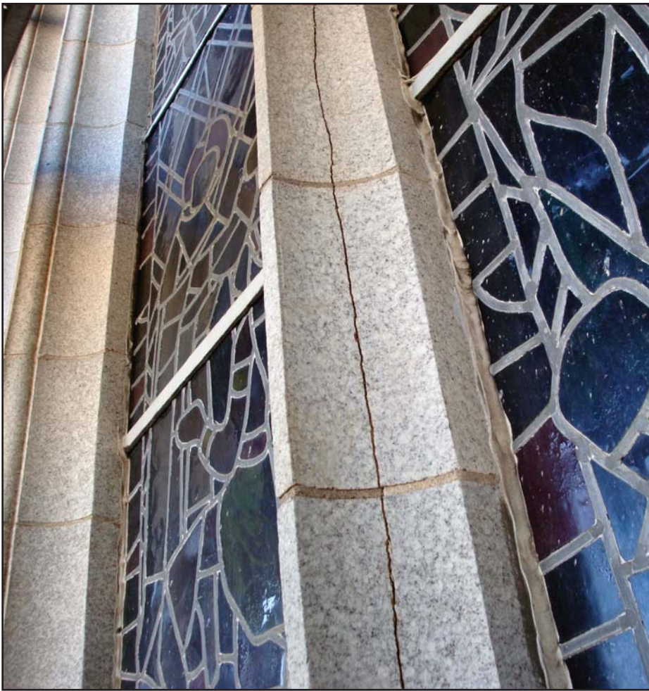
A vertical crack in a terra cotta mullion.
